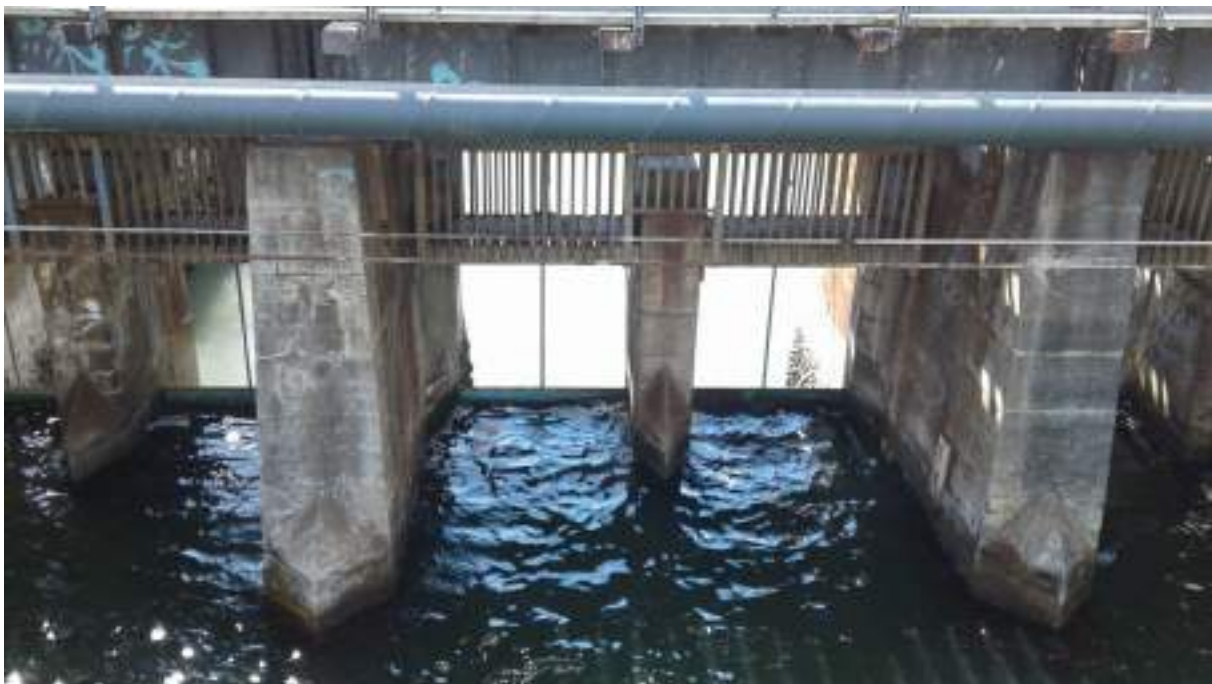
Figure 9 : The gates which control the water level of the Basin.
